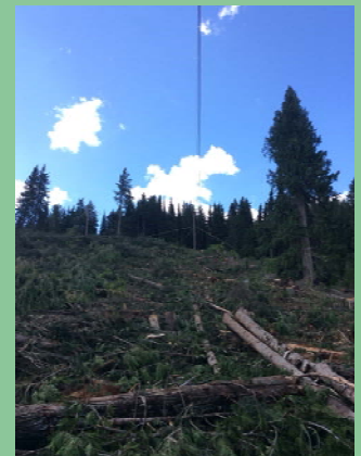
Photo of a typical cable yarding operation, with the photographer standing at the landing where the felled logs will be yarded to, and the cables visible against the blue sky. The single standing trees have been retained from harvest.
